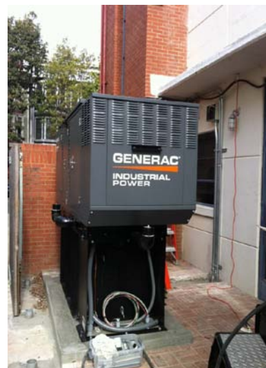
Fire Station #6 New Generator
