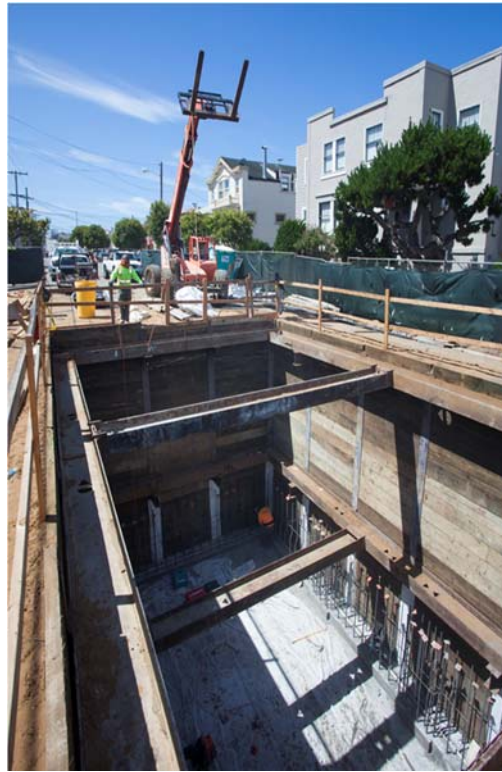
18th Avenue & Moraga Street cistern
