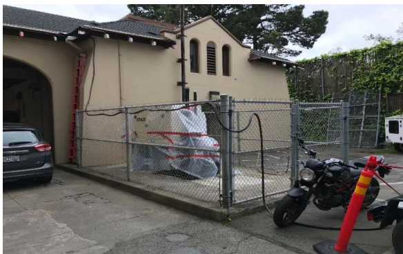
New generator and belly tank.
