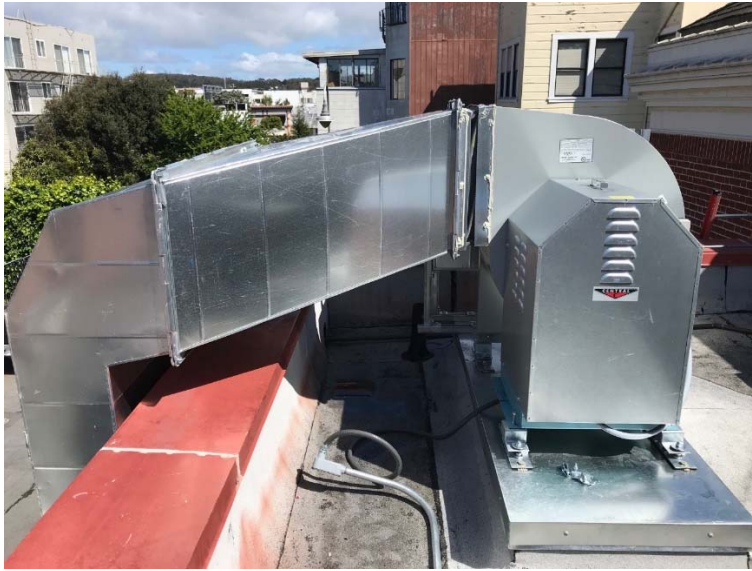
New roof-top supply fan.
