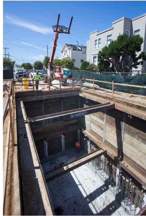
18th Avenue & Moraga Street cistern
