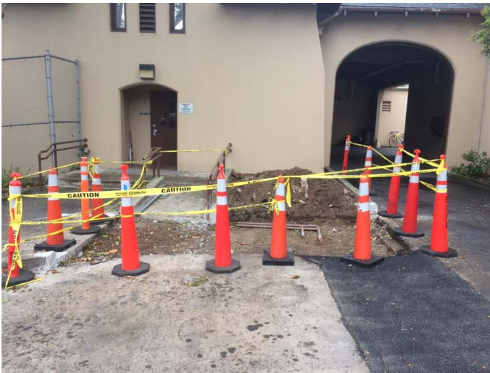
Ingleside Police Station – existing pavement being demolished, new accessible pedestrian path to the Community Room entrance will be constructed.
