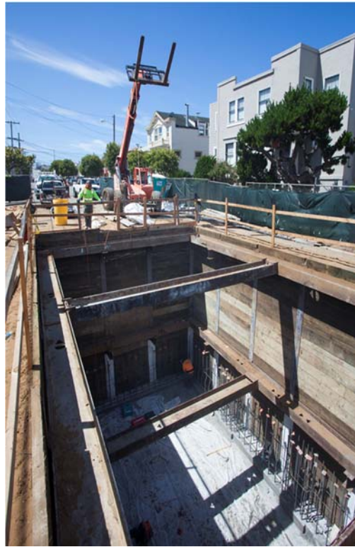
18th Avenue & Moraga Street cistern
