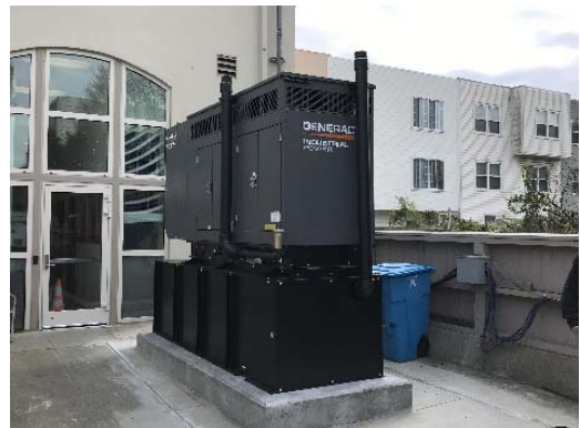
FS 31 – New Generator with 72-hr Runtime (February 26, 2020)
