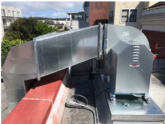
New roof-top supply fan.
