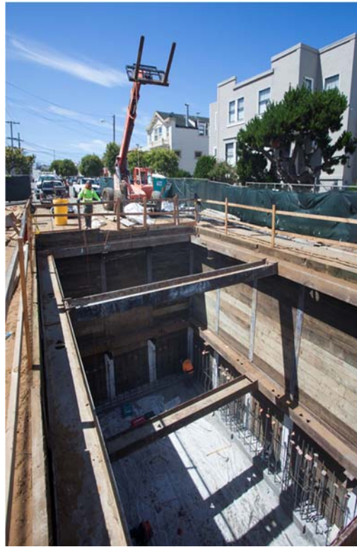
18th Avenue & Moraga Street cistern
