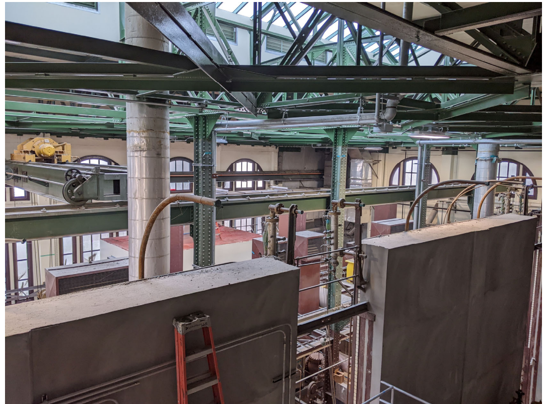
Pumping Station 2 at Fort Mason
