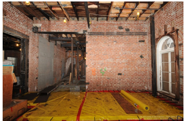
Interior of FS30 at Level 1
