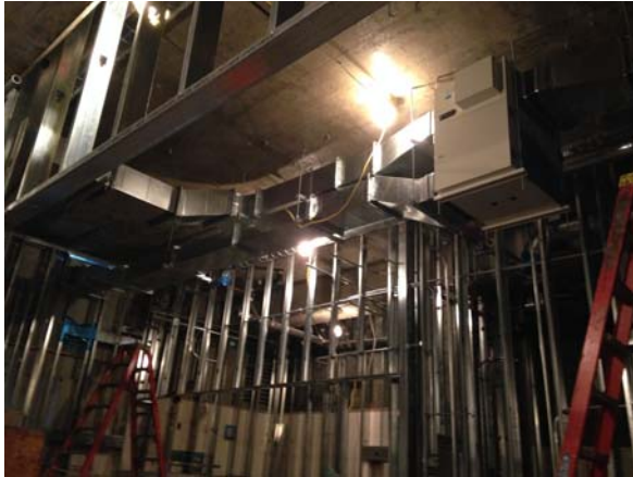
HVAC Duct Work
