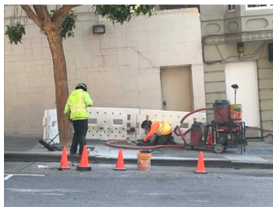
StreetTreeSF contractors remove tree-related tripping hazards from sidewalks in many locations through concrete slicing – a cost effective repair method that does not require removal and replacement of sidewalk squares.
