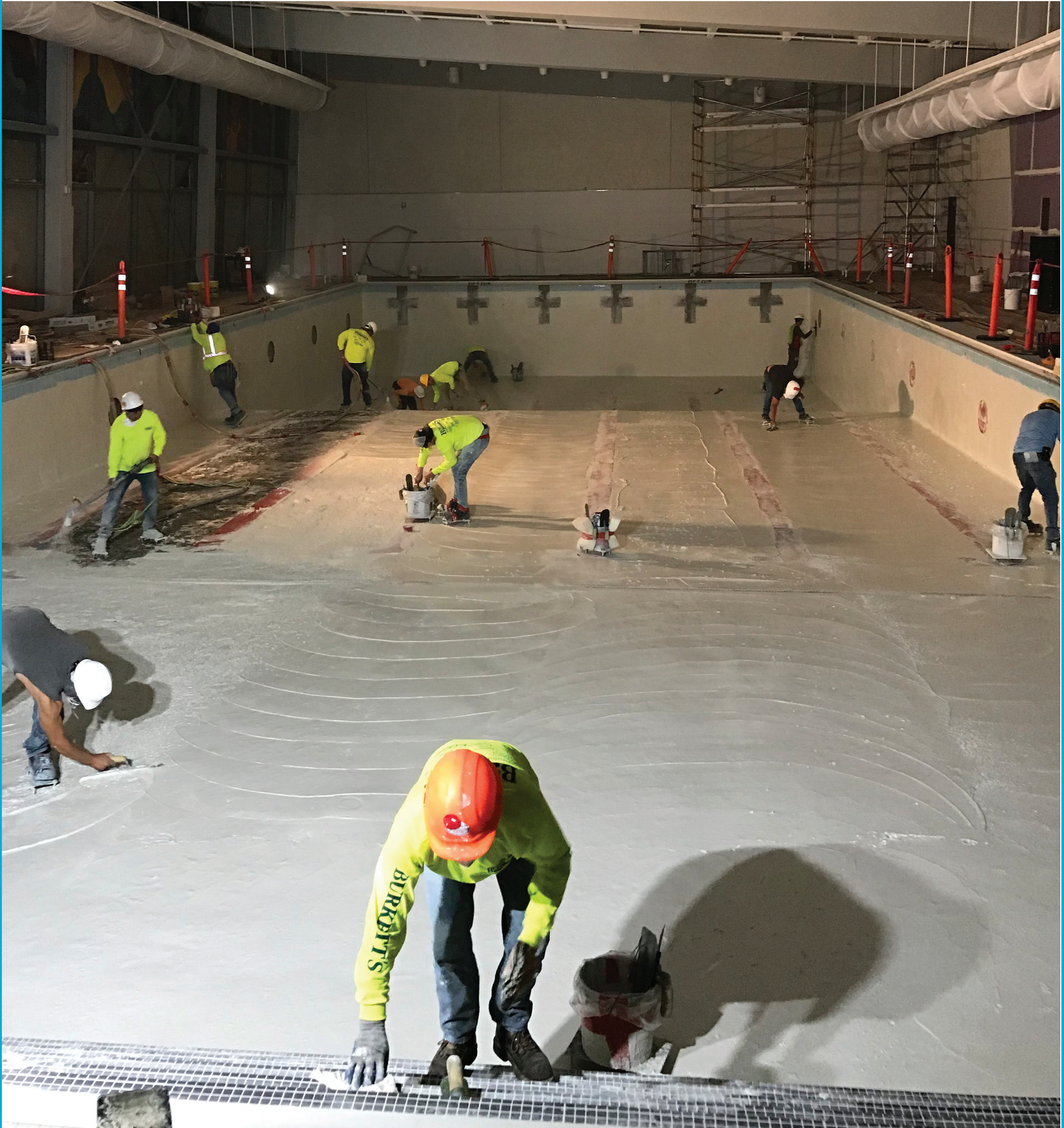
Plasterers work on Garfield Pool. The tricky part? To keep the water from seeping out, there can be no seams nor cracks. Photo by Jim Watkins
