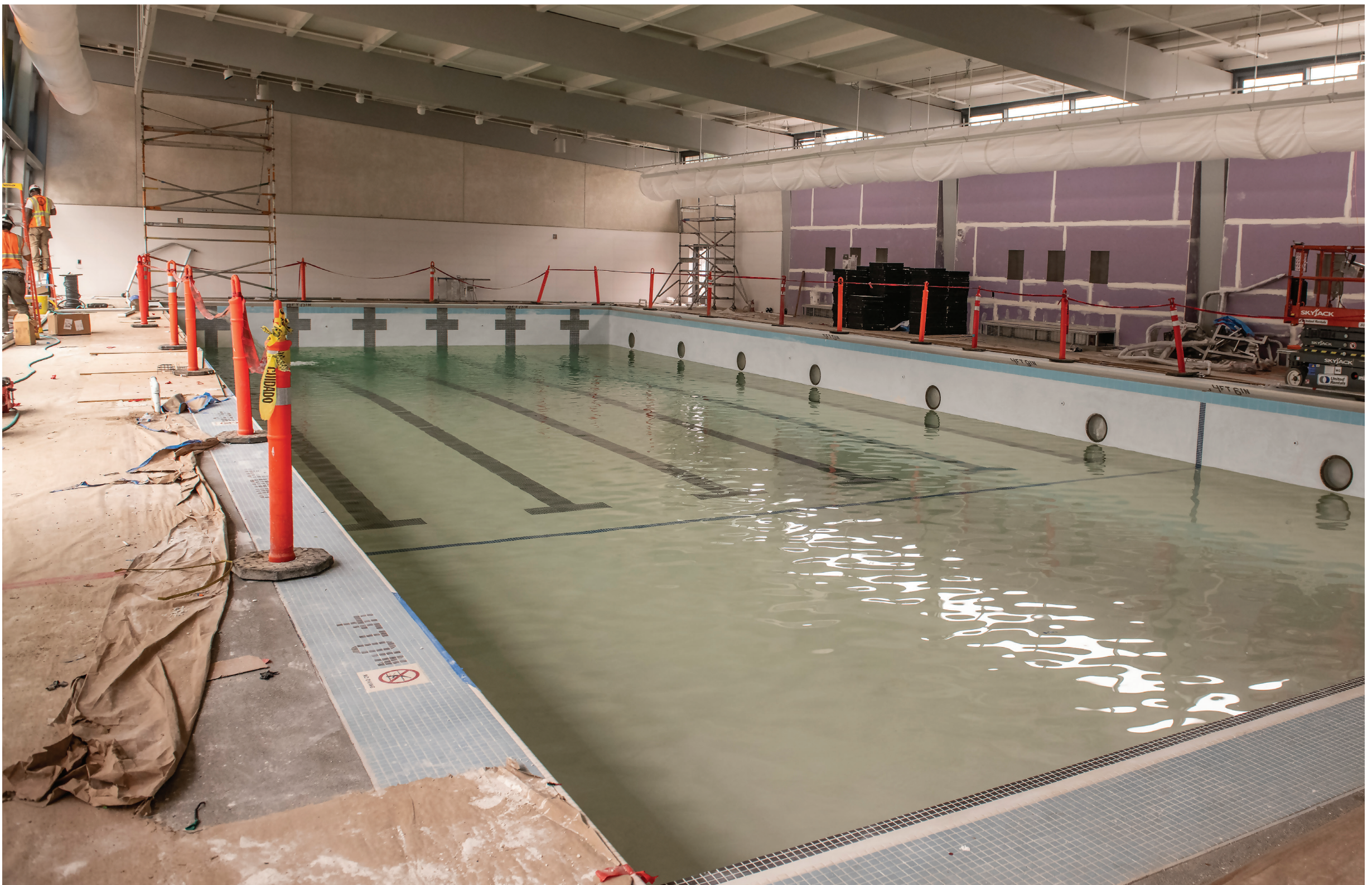
Once the plastering is complete, crews fill the newly lined pool with water. Photos by Jim Watkins
