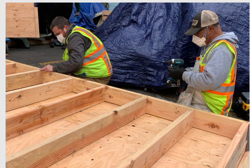
Screw by screw, crews begin to assemble platforms on site for immediate use.
