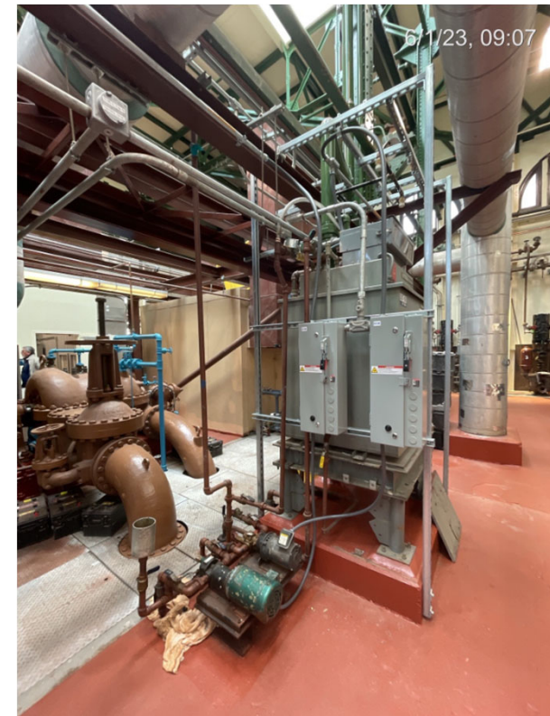
Pumping Station 2 at Fort Mason
