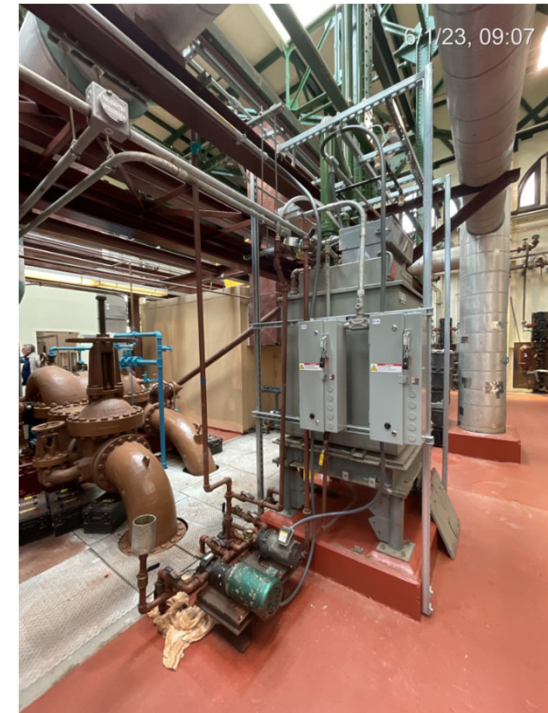
Pumping Station 2 at Fort Mason
