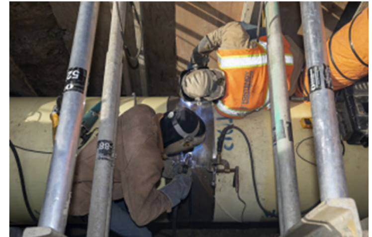
Installation of a new 36-inch (36") diameter welded steel pipe (WSP) at 19th Avenue and Sloat Boulevard
