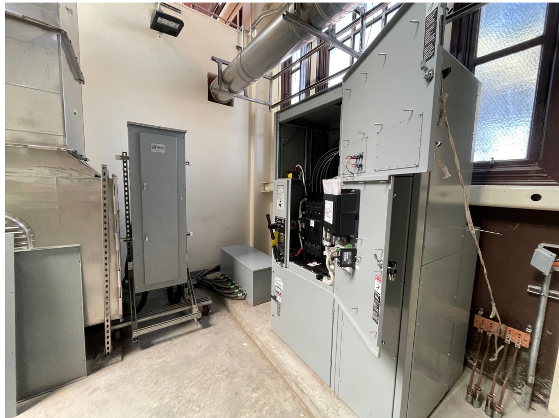
Pumping Station 2 at Fort Mason
