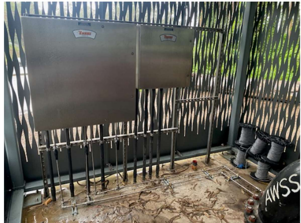
Clarendon Supply project: SCADA Unit
