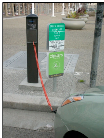
Electric Vehicle Charging Station
