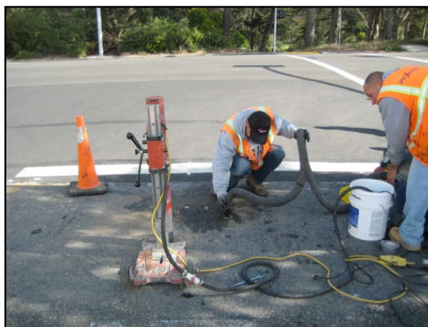
Staff installing new technology to improve traffic flows through the SFgo Project
