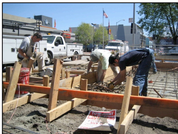
Crew Installing the Foundation for Two Backup Generators at the Hall of Justice
