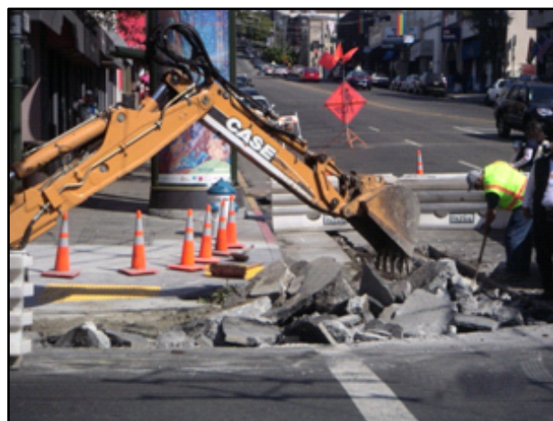
Crew Using Machinery to Dig and Trench Street to Repair Sewer Line
