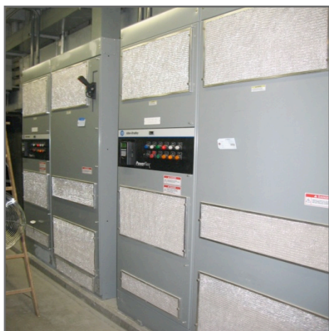
Newly installed control systems
