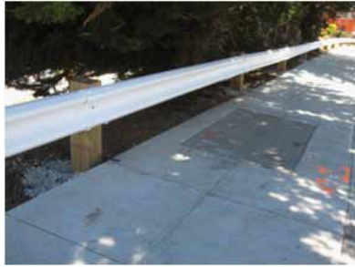
Bernal Heights Guardrail (before and after)
