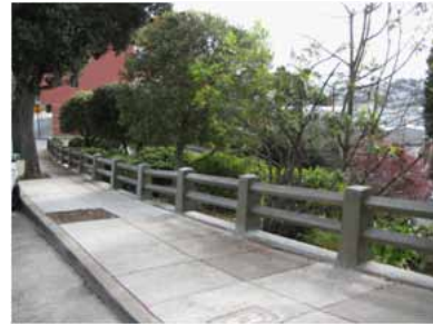
Roosevelt Way Guardrail (before and after)
