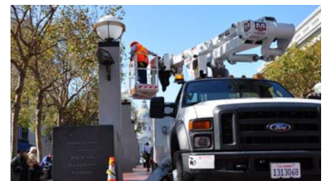
UN Plaza Re Lighting
